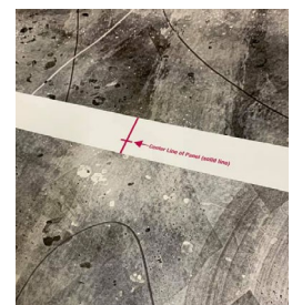
Shawn provided detailed notes of where the center of the panels were.
